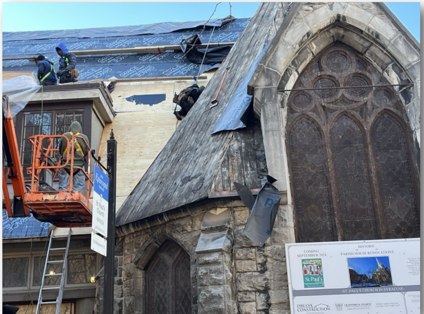
These brave workers have been completing the roof replacement in all kinds of weather!
